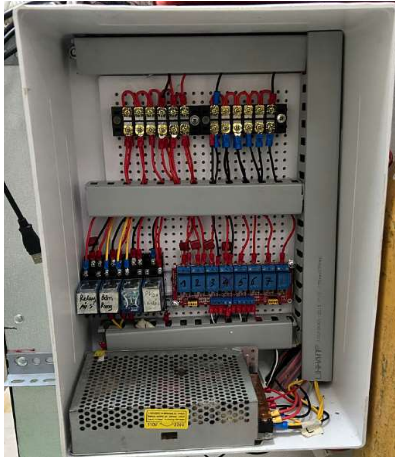
Figure 3.18 Electrical box of the machine
