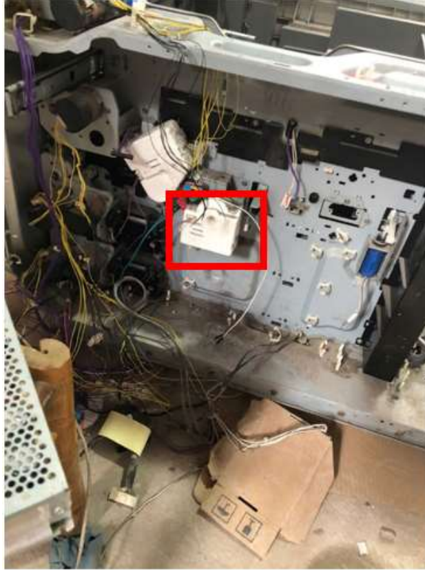
Figure 3.16 Actual installation positions of the motor
