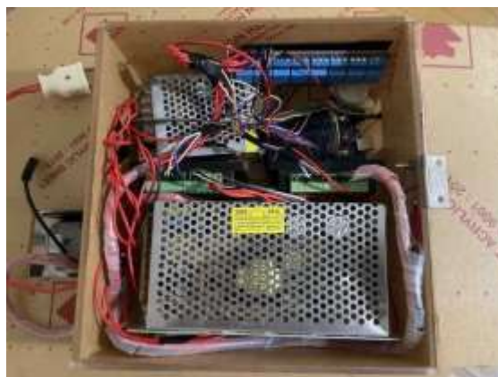
Figure 5.2 System electrical box
