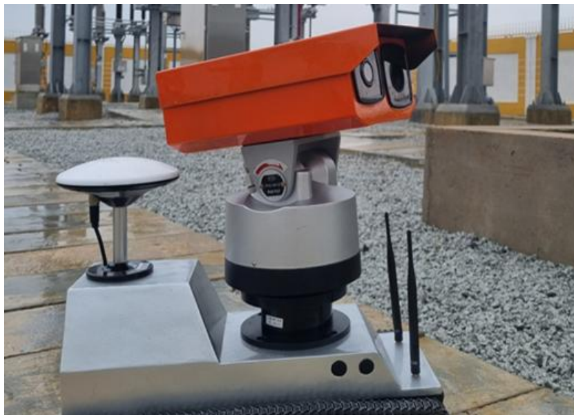
Figure 3: Substation monitoring robot
